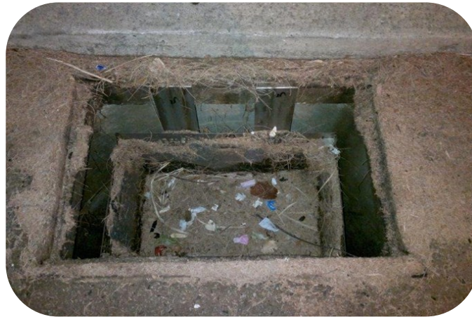
Figure 5: Stormwater drain insert to collect sediment
