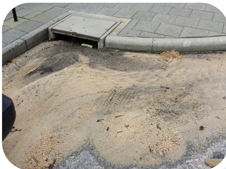
Figure 1: Build up of sand washing into side-entry drain
