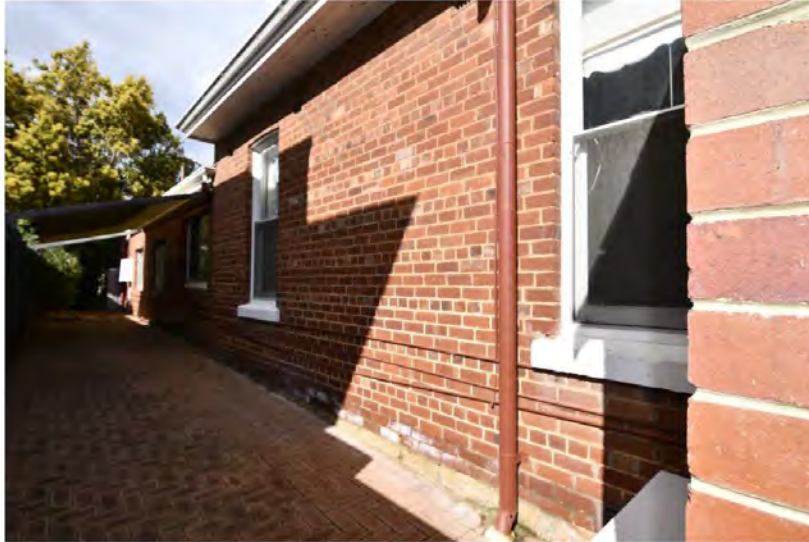
Photograph 9: The original east elevation in English garden wall bond and original windows. Griffiths Architects, September 2021.
