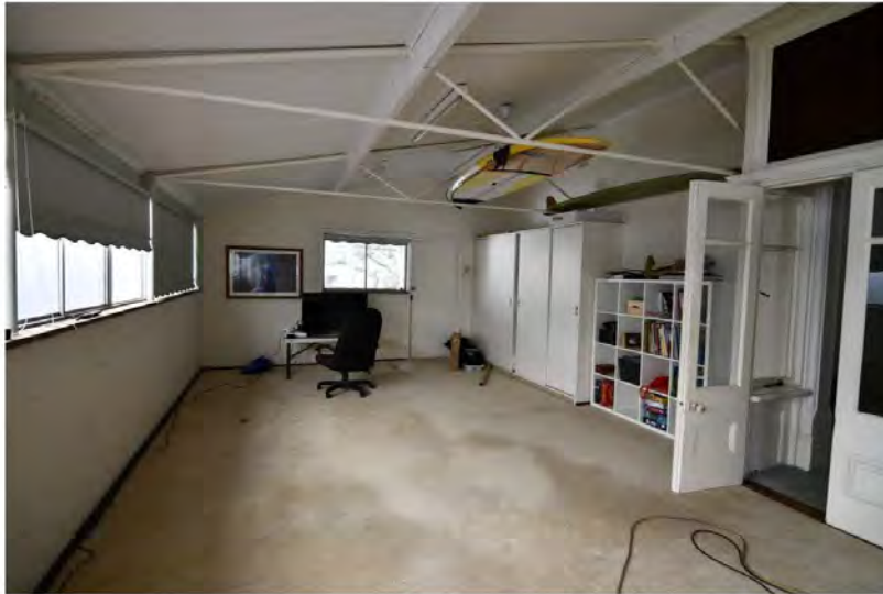
Photograph 18: The sleepout that shrouds the western elevation of the house with the dining room bay to the right. Griffiths Architects, September 2021.
