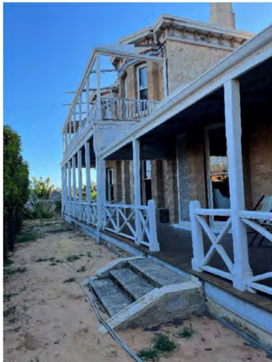
Photograph 04: Looking southwest showing the existing eastern verandah and double storey extension to the south. This fabric will be conserved and in part re-constructed and the single storey structure balustrade removed. Griffiths Architects, November 2021.
