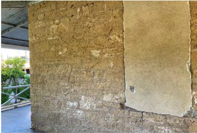
Photograph 01: Looking southeast towards a bricked-up window opening on the north façade. The window will be reinstated. Griffiths Architects, November 2021.
