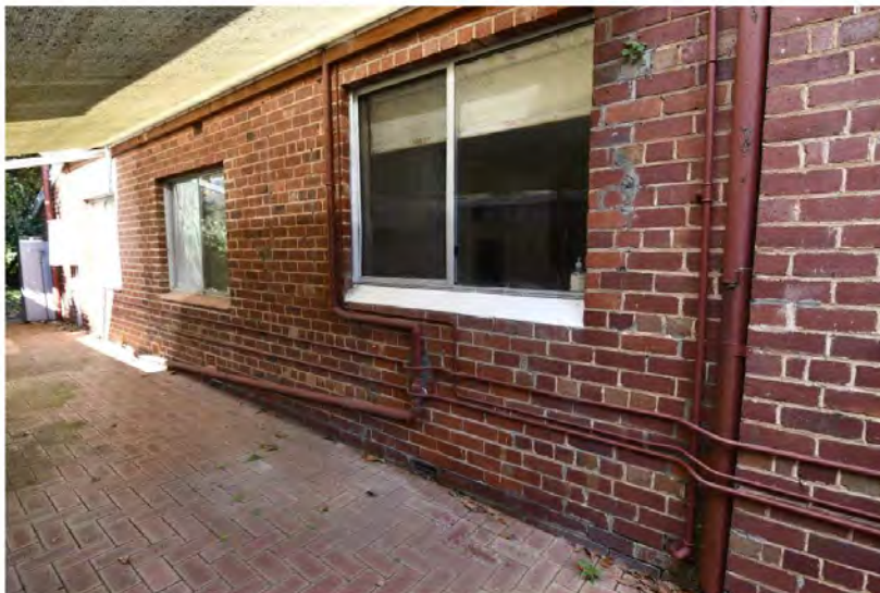
Photograph 10: Original brickwork from the first kitchen with later bedroom and laundry additions beyond. Griffiths Architects, September 2021.
