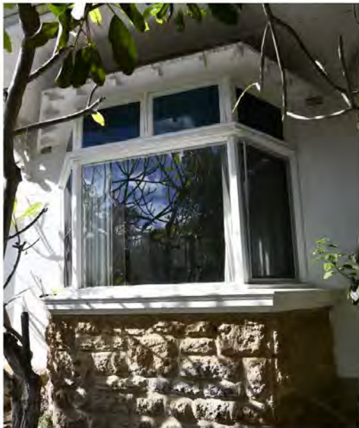
Photograph 8: The bay window, indicating two sashes removed to make way for the fixed pane. Griffiths Architects, September 2021.
