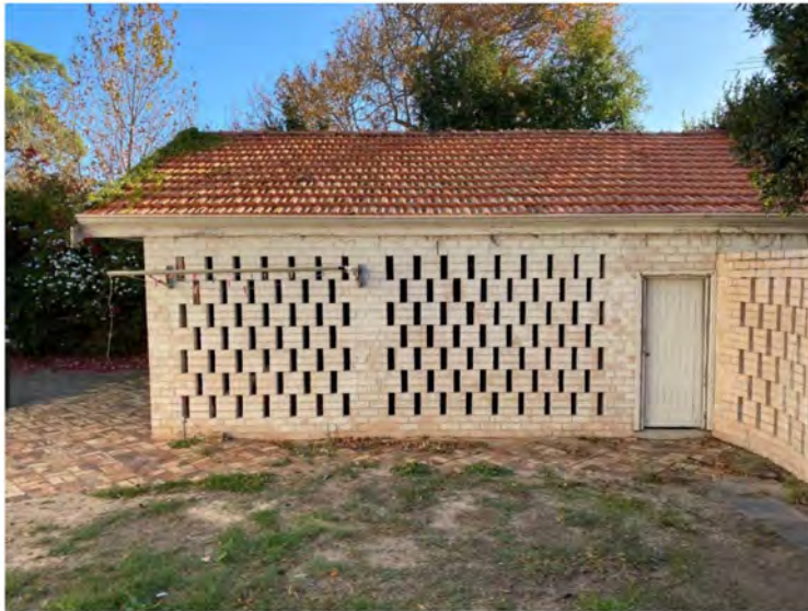
GARAGE | VIEW LOOKING WEST INCLUDING EDGE OF CURVED WALL TO BE REMOVED
