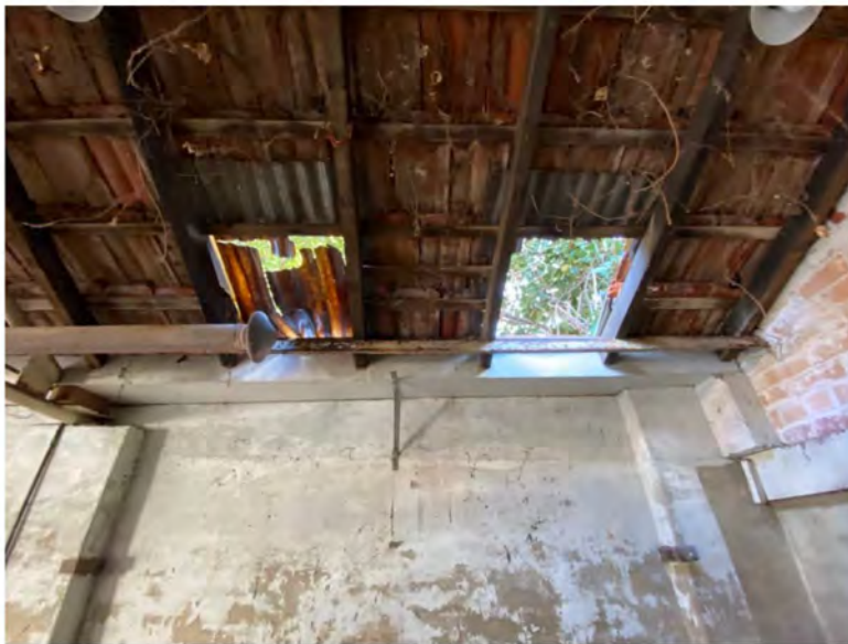
GARAGE INTERNAL | VIEW LOOKING WEST DAMAGED ROOF
