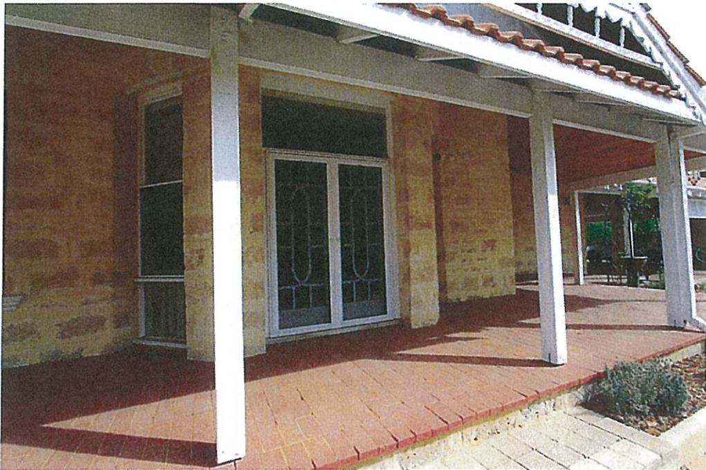
This room is an addition, infilling an original open area and access to the basement.
