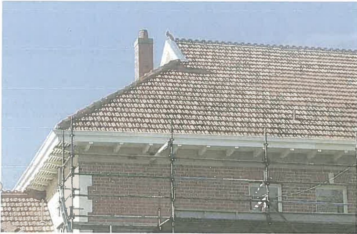
Figure 2: Existing Marseille profiled clay roof tiles, finial and ridge capping of the main house
