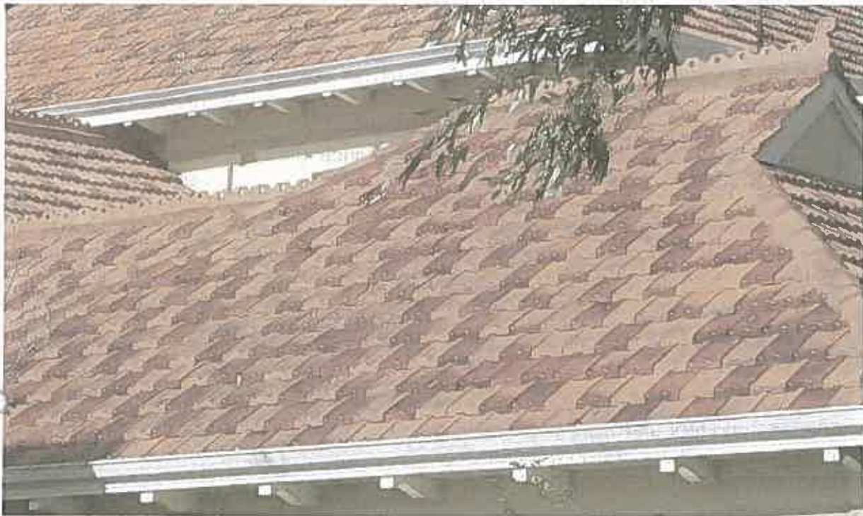
Figure 5: Sample of contemporary glazed terracotta Marseille files on the 1999 / 2000 garage addition, with a mix of glazed and unglazed files, gradation in colour to replicate the characteristic hues of the historic tiles. The gradation are uniform and the glazed finish are not consistent with the historic tiles on the main roof.
