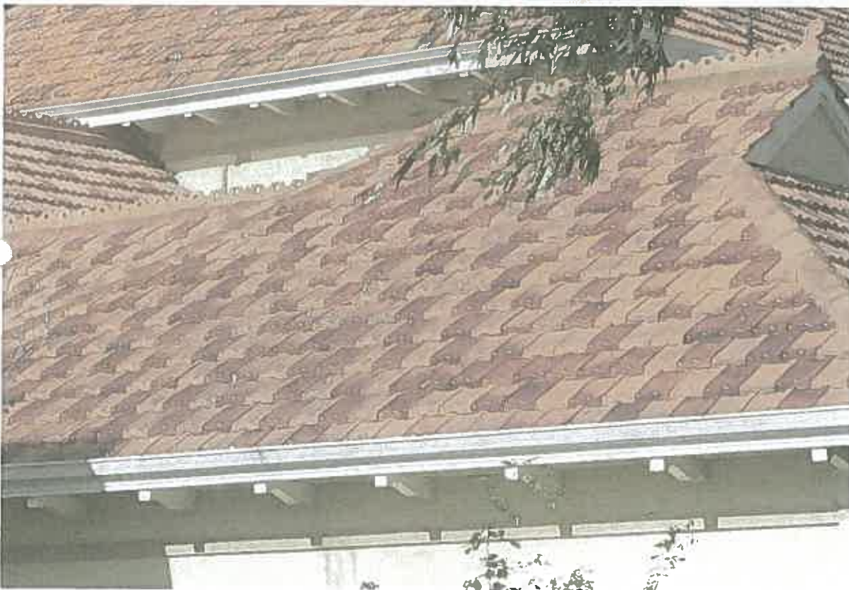
Figure 3: Existing Marseille clay roof tiles, a mix of glazed and unglazed files, of the circa 2000 addition
