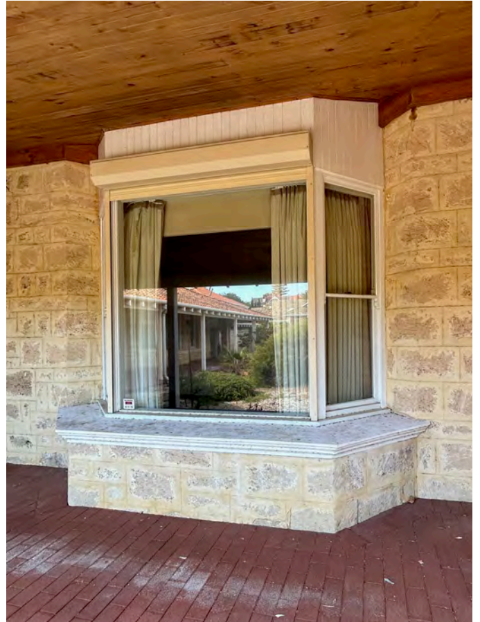
Image 36. View east of bay window to western facade of 1986 southern extension. (Source: PA 2023)
