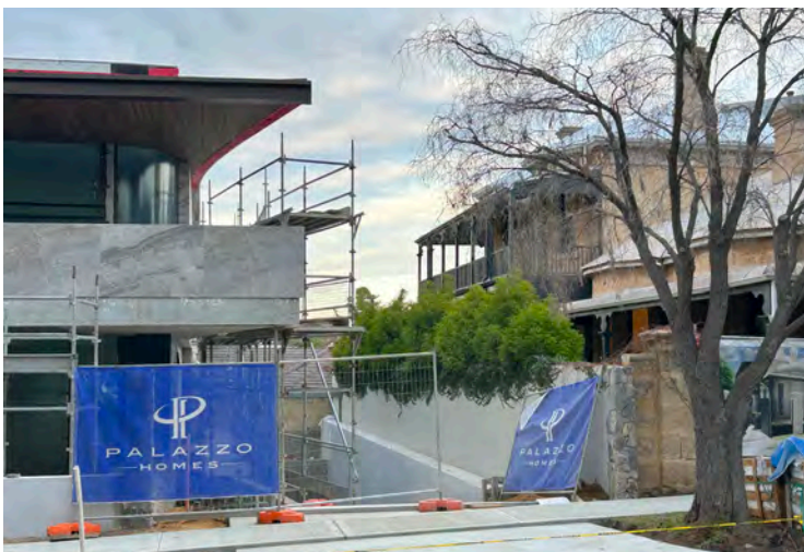
Image 111. View south capturing the new boundary between 72 Leake Street and the new residential development on The Esplanade. (Source: PA 2023)
