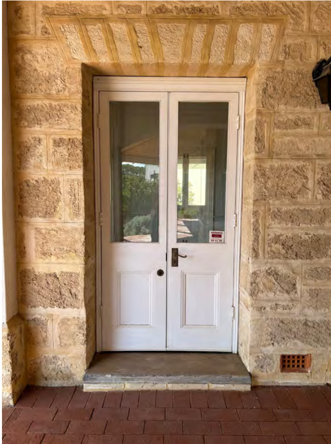
Image 22. Detail image of northern double door to 1927 'Dining Room'. Note difference in stone lintel to the rest of wall. (Source: PA 2023)
