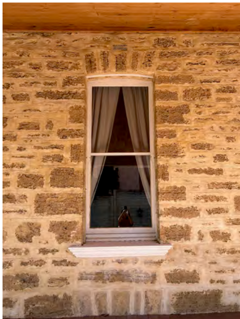
Image 15. Detail image of original 1897 timber hung window to north facade. Note stone lintel below window, indicating an opening (window or door) to the cellar below that is no longer accessible. (Source: PA 2023)
