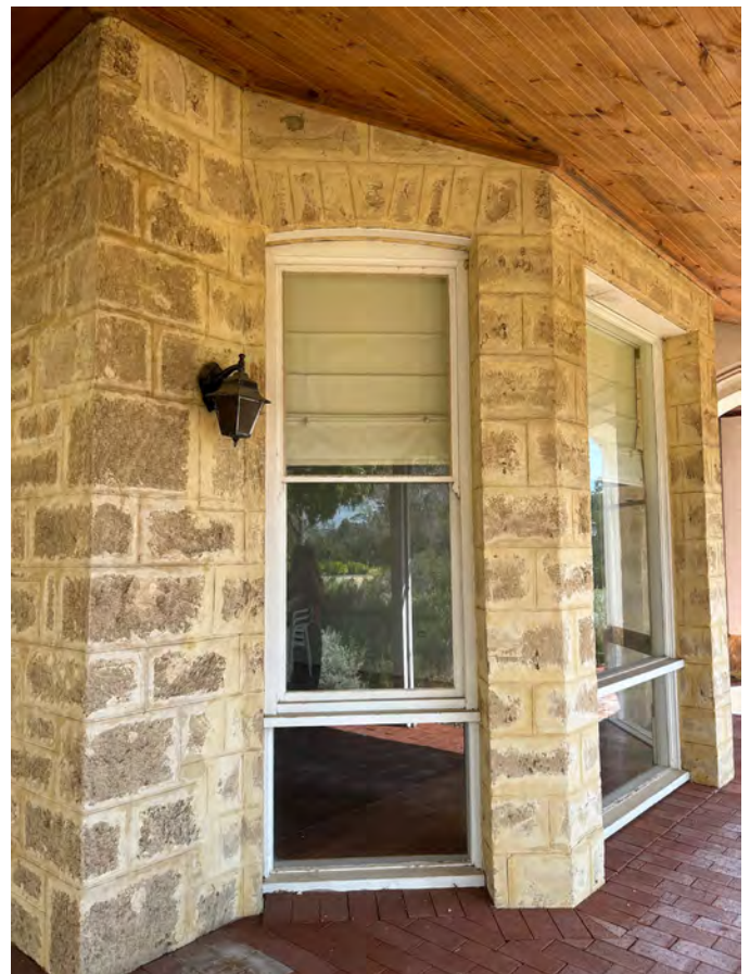
Image 24. View north towards 1986 bay window addition to 1927 'Dining Room'. Note transition from Cottesloe to Carabooda limestone. (Source: PA 2023)
