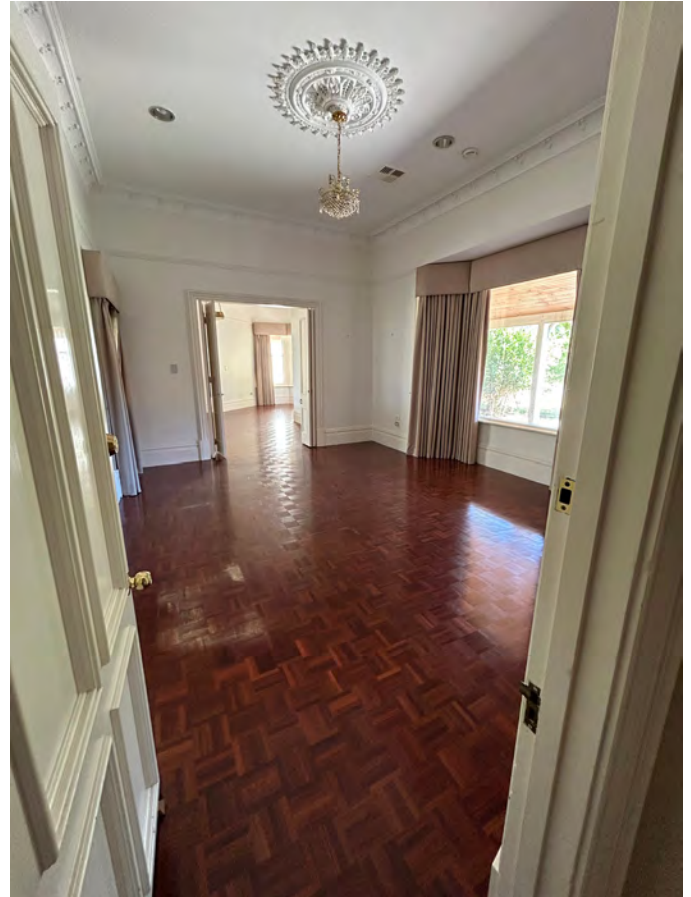
Image 102. View south into 1986 Lounge and Bedroom addition. Note parquet floor, timber skirting, ceiling rose and cornice and shallow bay window. (Source: PA 2023)
