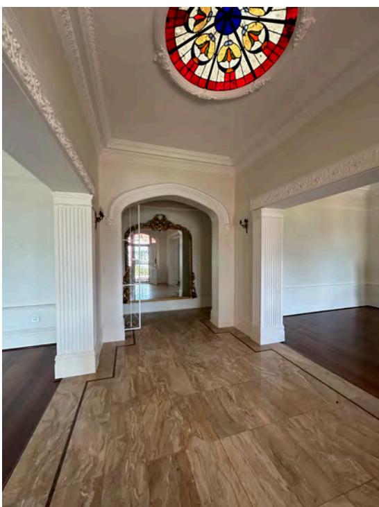
Image 55. View west from main entry door towards main corridor, capturing skylight from 1986 build. (Source: PA 2023)
