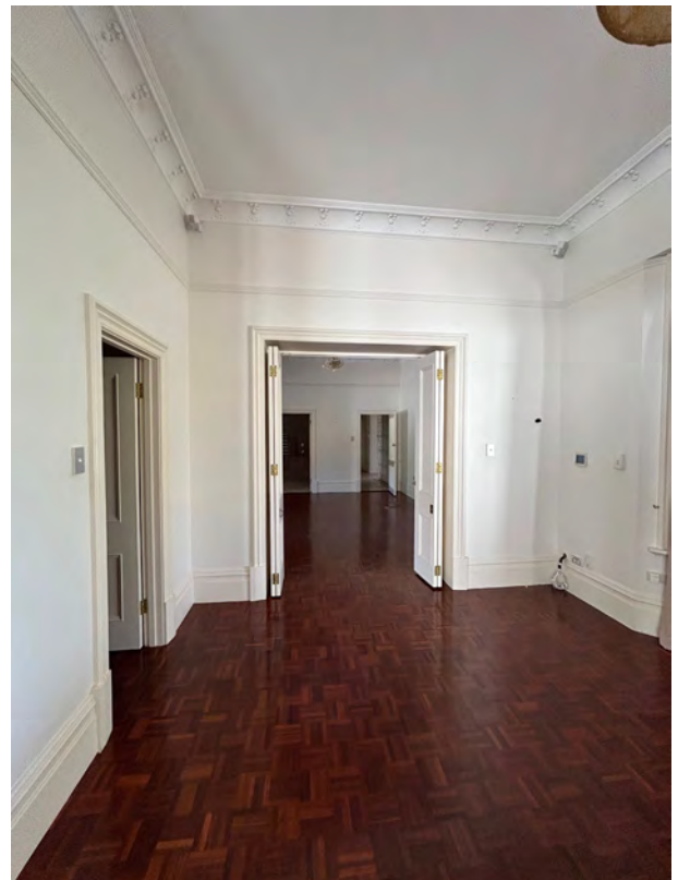
Image 108. View north from southern Bedroom into Lounge of 1986 addition. Captures walk-in-robe and timber skirting and decorative ceiling mouldings. (Source: PA 2023)
