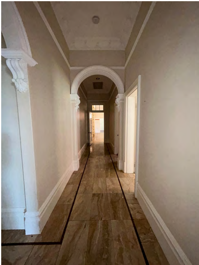
Image 74. View west from eastern end of corridor towards Bathroom and Lounge Room, capturing both archways, timber skirting and stone tile flooring. (Source: PA 2023)
