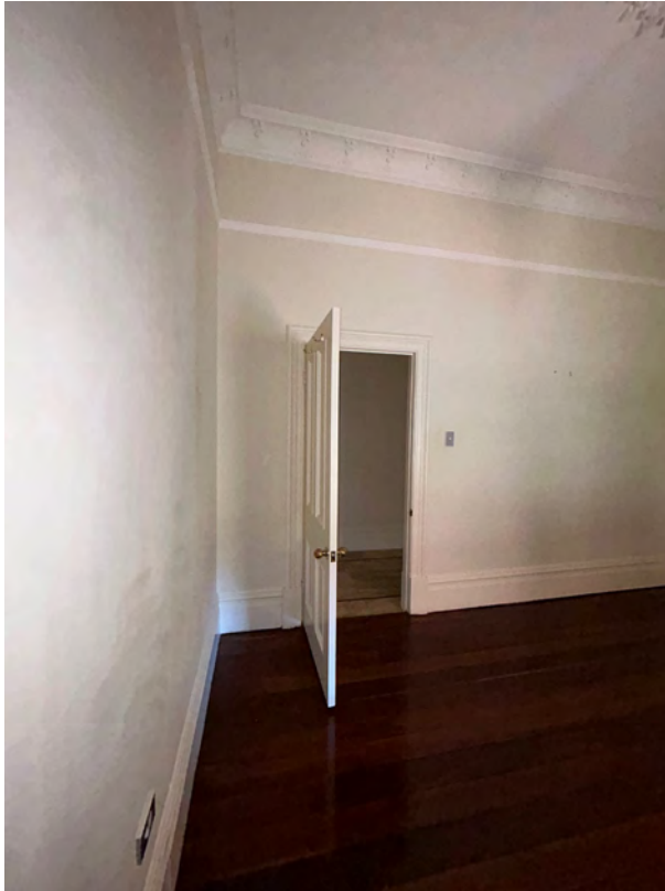
Image 79. View south towards Bedroom door. Capturing early timber floor and skirting and decorative ceiling cornice. (Source: PA 2023)
