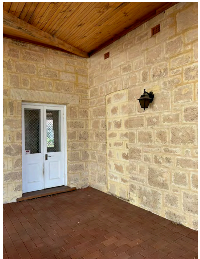
Image 27. Detail image of south-west external corner of 1927 'Dining Room'. Note difference in stone lintel to existing door, and infill to former door opening. (Source: PA 2023)
