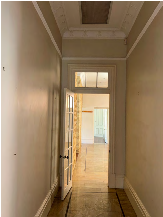
Image 81. View west down corridor towards Lounge Room off Kitchen. Capturing timber door with toplight. (Source: PA 2023)
