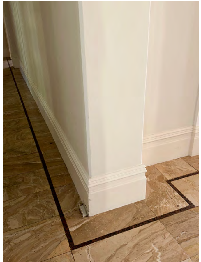
Image 69. Detail image of timber skirting and stone tile flooring to Entry Hall and corridor. (Source: PA 2023)
