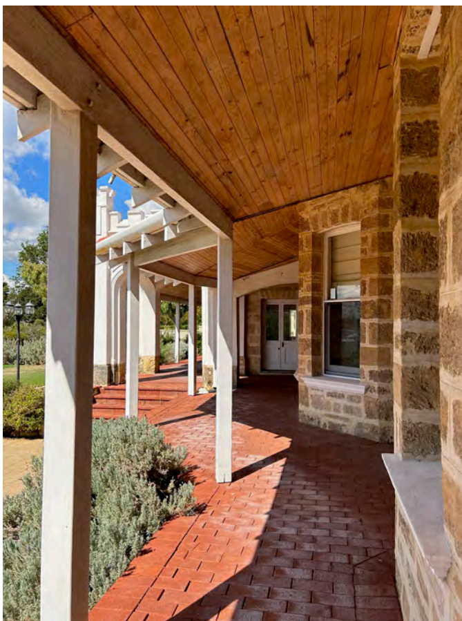
Image 21. View south along front (east) verandah from northern corner of 1897 fabric towards 1927 fabric. Note contemporary brick paved verandah, squared timber posts and timber ceiling lining. (Source: PA 2023)
