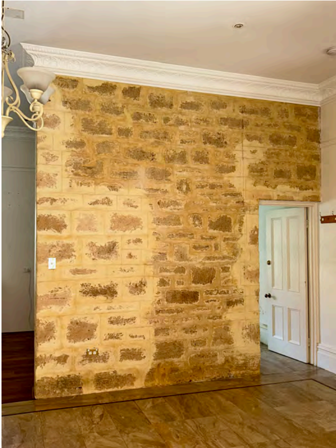
Image 87. View south from within Lounge Room towards Laundry. Note patching to limestone wall. (Source: PA 2023)
