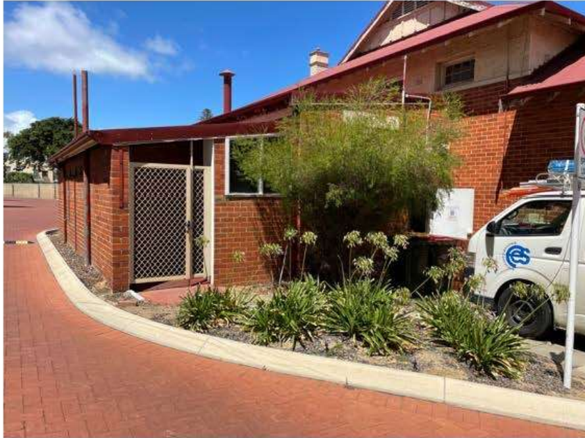
Photograph D4: The toilets at the rear which are intrusive. They have been modified, added to ad no longer meet NCC requirements. Griffiths Architects February 2022
