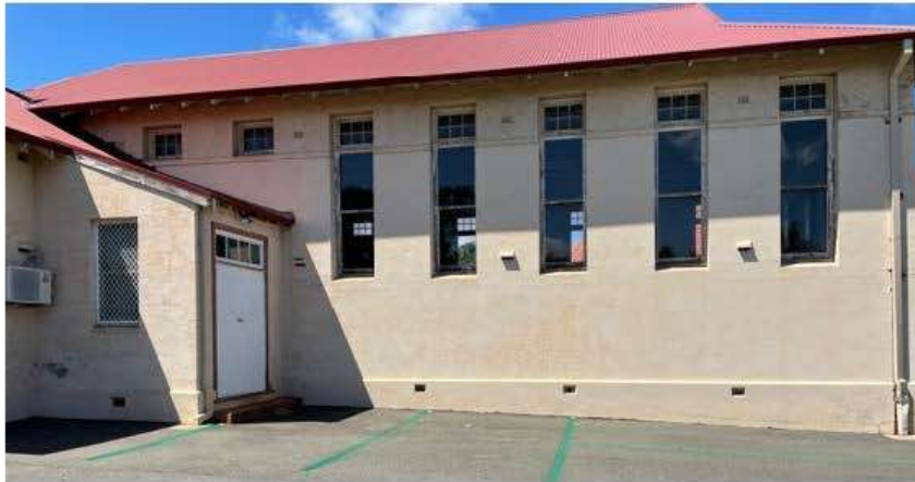
Photograph 03: North elevation showing similar deterioration. Griffiths Architects February 2022
