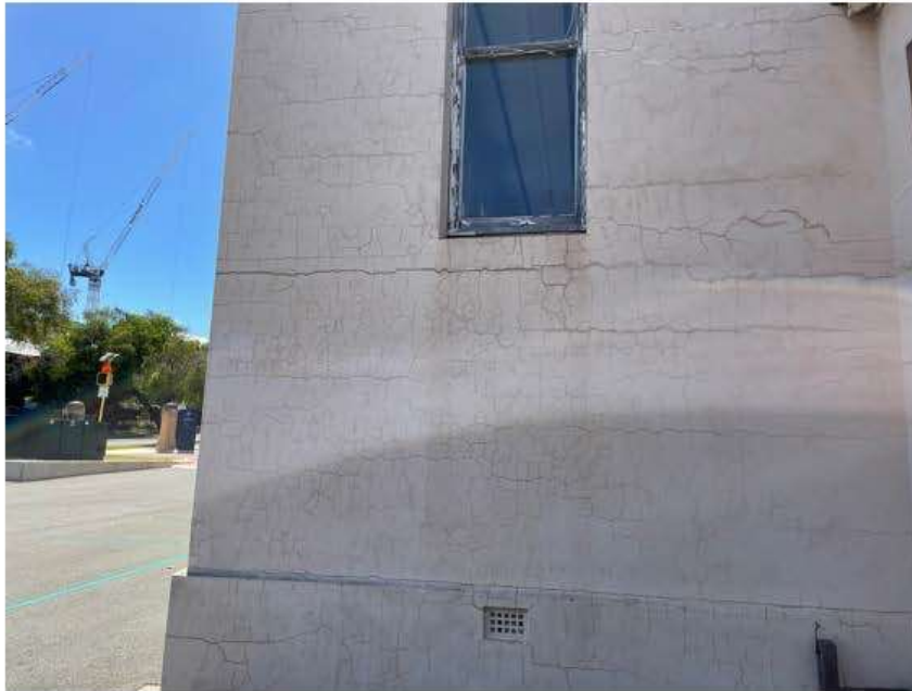
Photograph 02: Poor state of the rendered walls and joinery. Griffiths Architects February 2022
