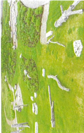
WSUD with broken kerb
