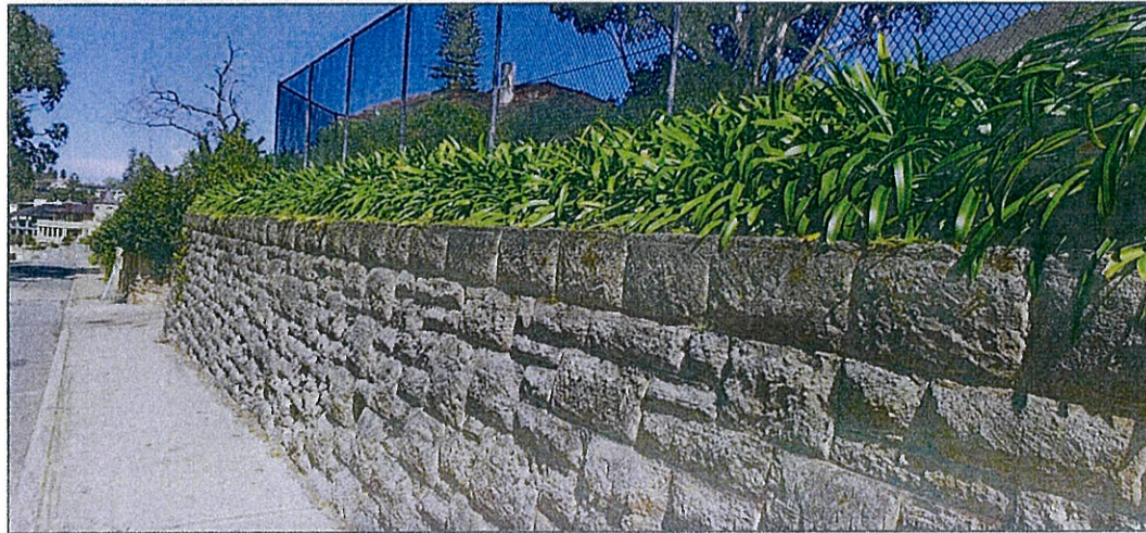
Photograph 4: The solid wall of No.22 The Esplanade. The sloping site has been levelled out, with a high wall on the southern boundary.
