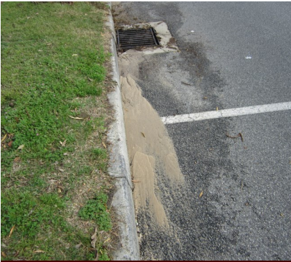
Sand drift into drains
